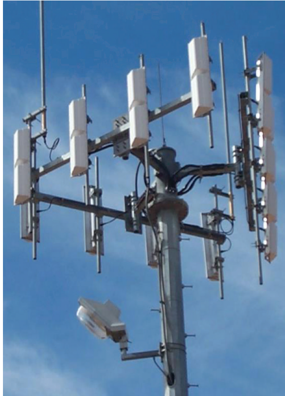
Figure 4.26 Triangular array of dipoles used as a sectoral base-station antenna for mobile communication.
